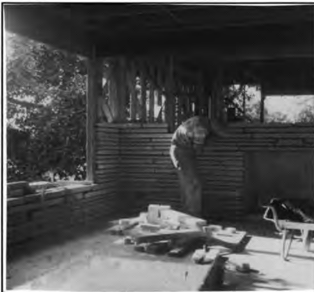
Bob Van Tuyl meticulously constructs the centerpiece of his dream house - a fireplace wall of flagstone. He would later install plate glass in the opening on the left, to enclose an indoor planter.
